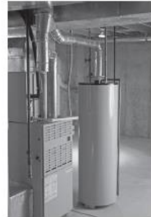
Heating systems (© Comstock RF.)
