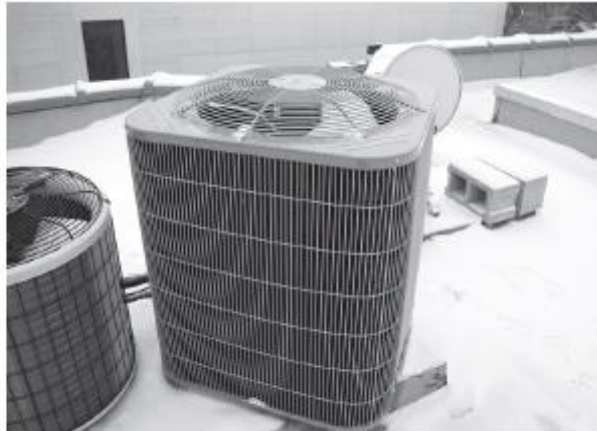
Air conditioning systems (© The McGraw-Hill Companies, Inc./Jill Braaten, photographer.)
